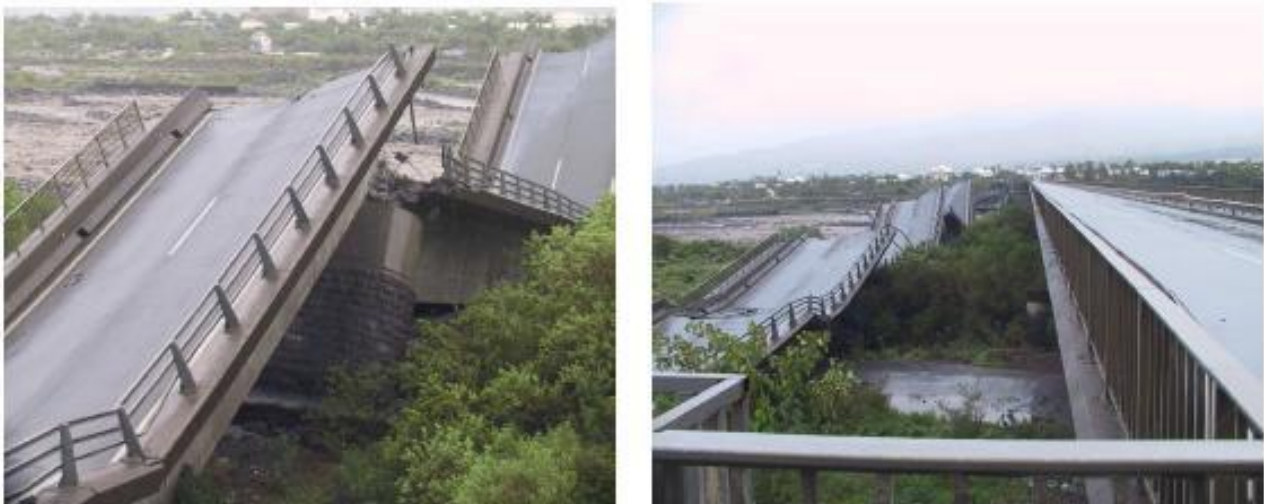
Figure 21: Photos of a bridge on the Saint-Étienne River on Réunion Island, which collapsed on 26 February 2007, when Cyclone Gamede hit Réunion. The cyclone was accompanied by heavy precipitation, which eroded certain piles and caused several spans to collapse. Source: DDE La Réunion.
