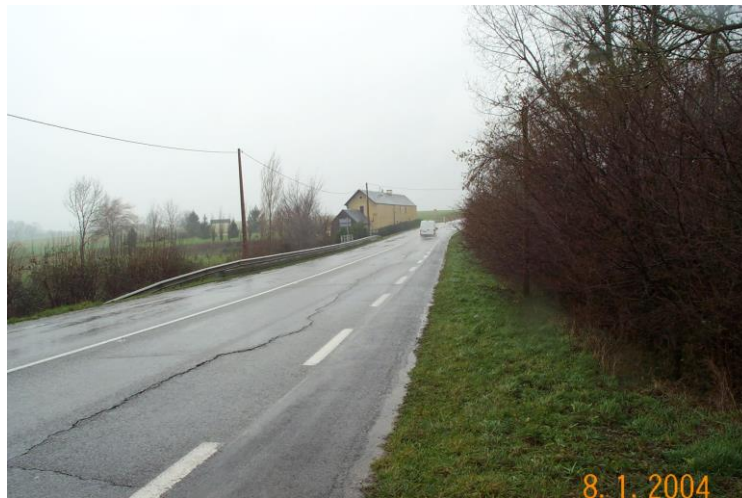
Figure 18: Photograph of fill on the RN158 in Macé, France, in which the cracks and settlements became worse after the summer of 2003. Source: Cerema, DTerNC.
